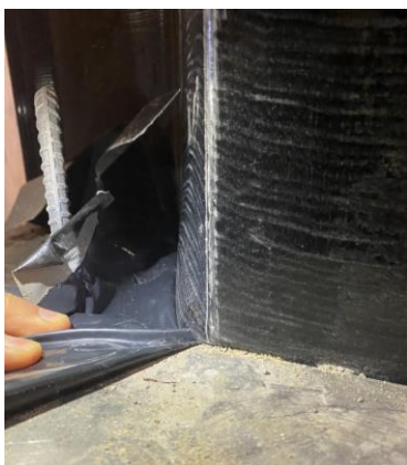
Fig. 20. Buckling about weak axis.
