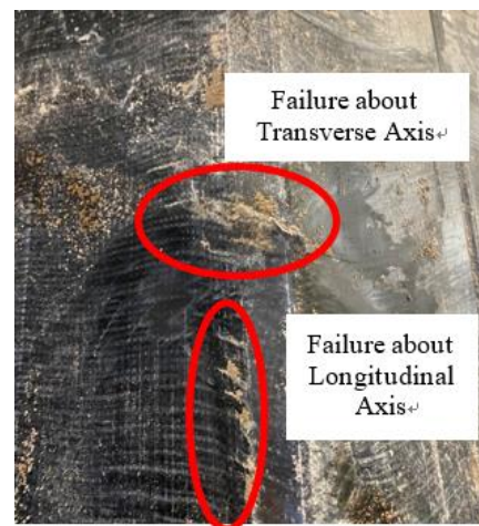
Fig. 26. Sheet pile failure.
