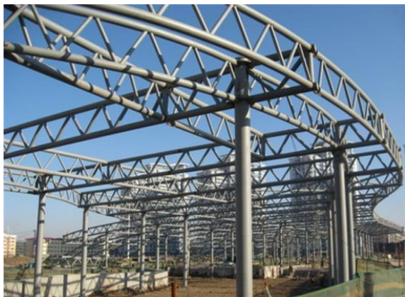
(a) Steel tubular truss at a station building in Jiangsu Province, China
