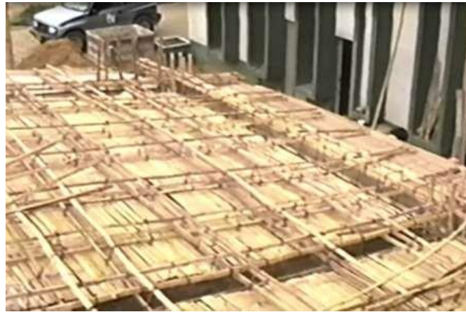
Fig. 12. Formwork for roof slab with the use of chopped Guadua cane, wooden quarters, round cane shoring, slab reinforcement with Guadua cane slabs and 6mm stirrups of the same material [34, 44, 46].
