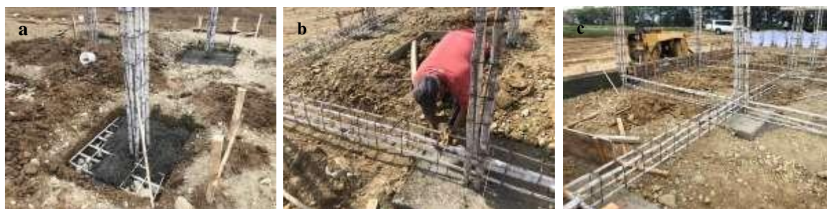
Fig. 10. Foundation preparation: a Construction of plinths and columns, b Placement and rectification of bracing walls, c Casting of the footing beam with lightweight concrete with rice husk.
