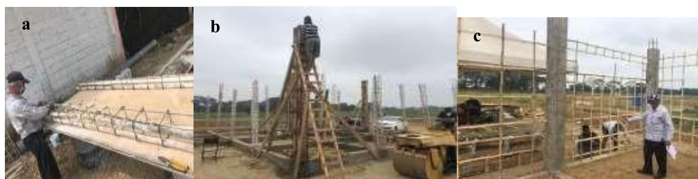
(a) Construction of the structure (b) Formwork (c) Column cast with hybrid light concrete
