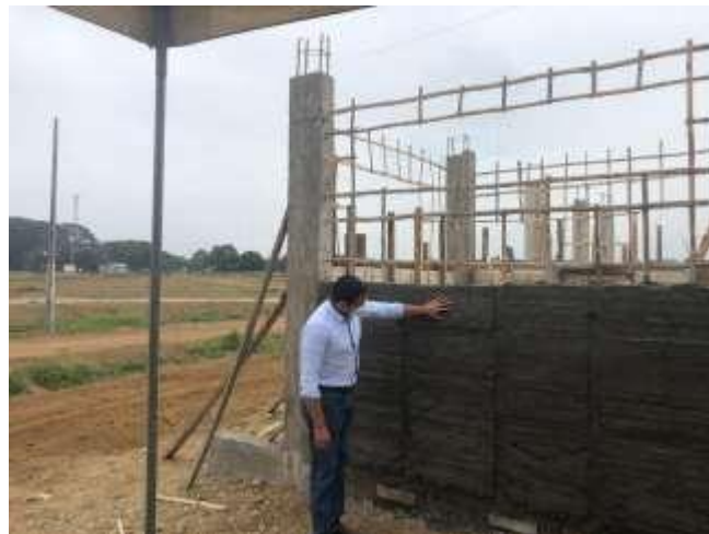
Fig. 13. In situ construction of the walls with hybrid lightweight concrete with rice husk and Guadua reed lattice. Based on the ancestral technique of bahareque or tapial.
